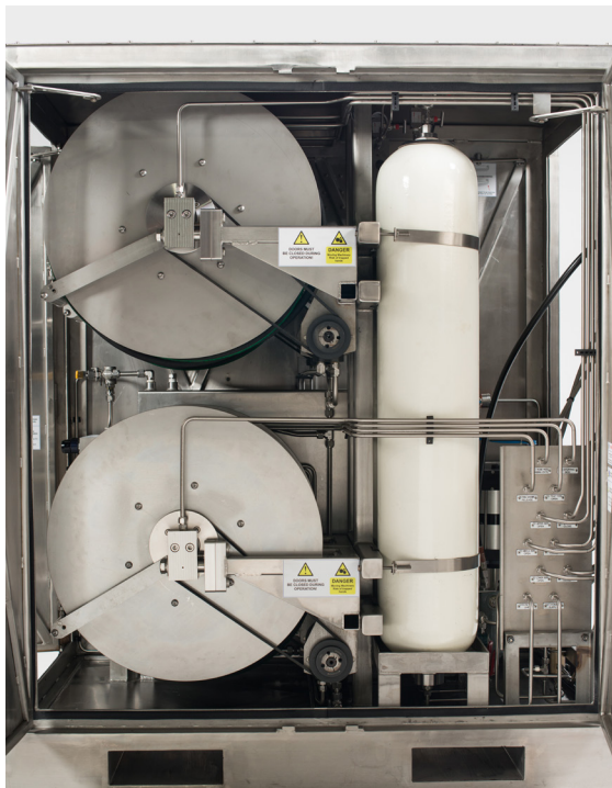
Hydraulic Motor reels within Phuel Pressure Control Unit
